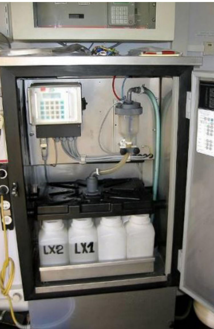
River water collectors installed in containers of TELERAD river beacons
